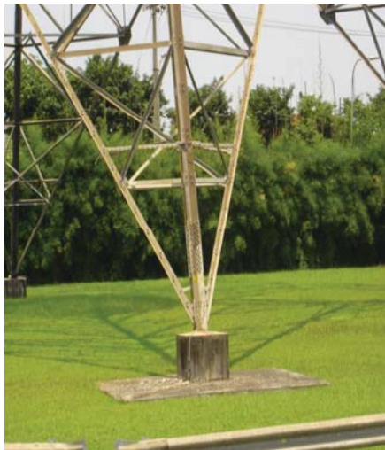
Gambar 4.15 Pondasi tower (lattice) SUTET 500 kV Gresik - Krian
