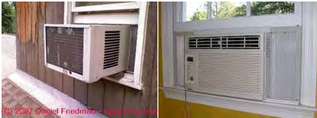
Gambar 6.2 Instalasi AC Window
